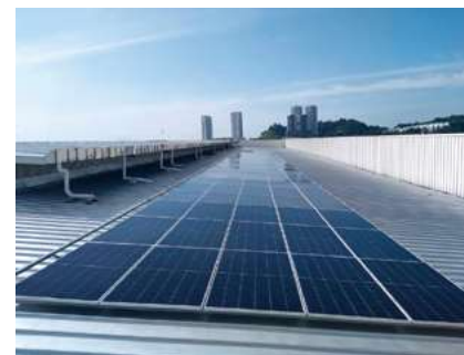
Penang Logistics Center solar panels
