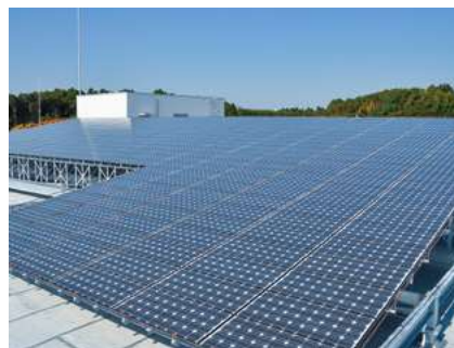
Narita Terminal solar power generation
