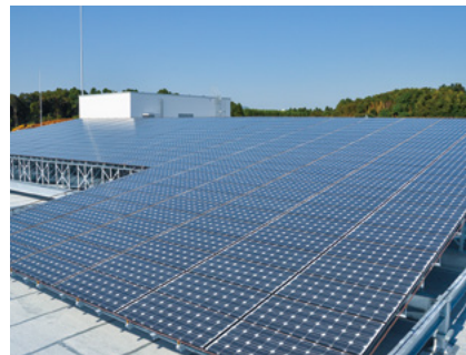
Narita Terminal solar power generation
